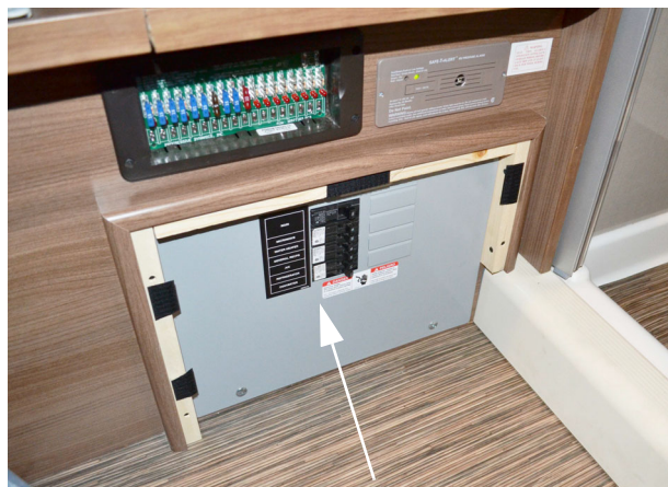
120-Volt Circuit Breakers -Typical View
