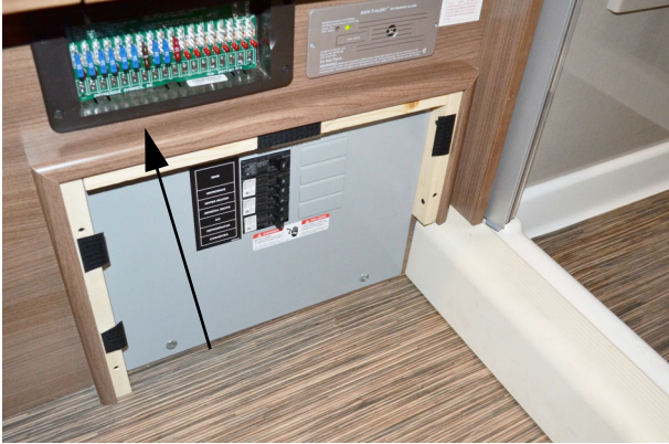
House 12-Volt Fuses (Located on right side twin bed cabinet at rear) -Typical View
