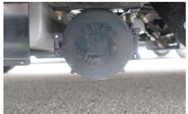
Sewage Drain Hose (Located beneath left sidewall) -Typical View
